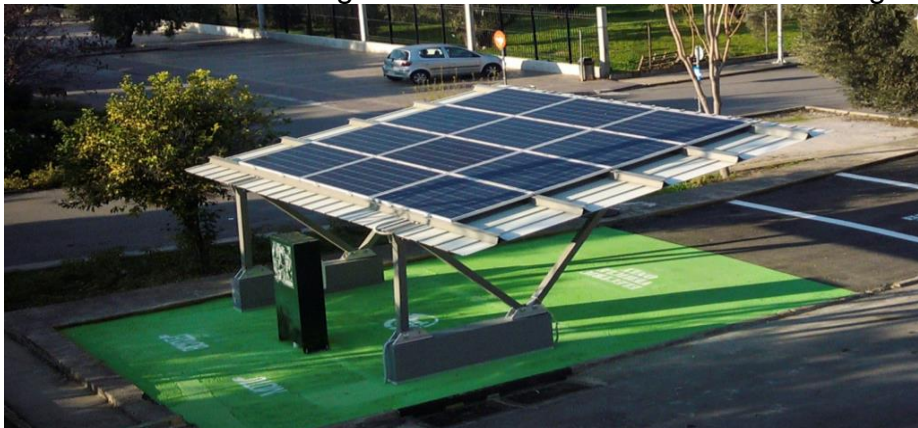
Fig. 9. PV-battery ev carport
